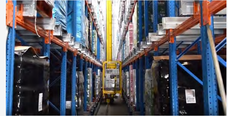
Automated Racking Systems
